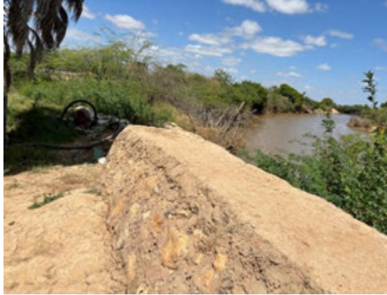
Sigalow – Yusuf A site in Beledweyn: A gap at the end of masonry wall
