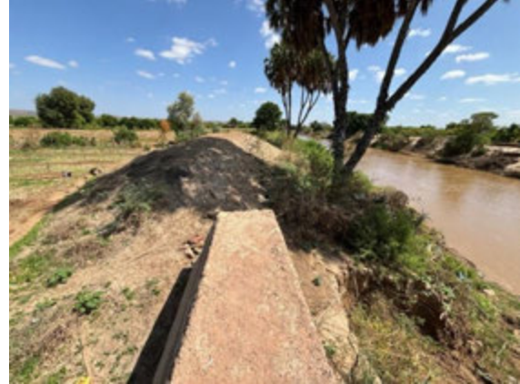
Hawatako 4 site in Beledweyn: A gap at the end of masonry wall
