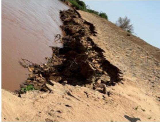
A portion of the stone pitching is washed away by floods in Sulgudud 1 site Dolow
