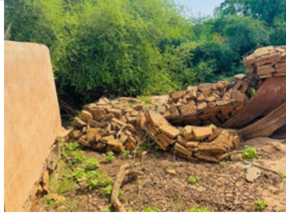
A portion of the gabion wall is collapsed Sulgudud/Hussein site Dolow
